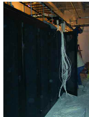
The reduction in cabinet requirements allowed a design change in how they were laid out.
